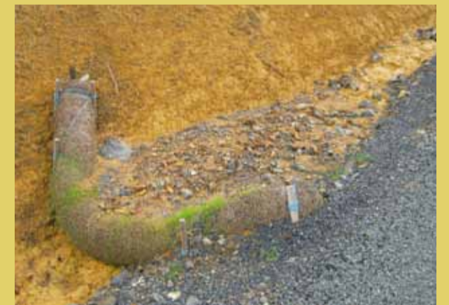
Straw Wattles make extremely effective check dams allowing water to pass through whilst trapping material on the upside.
