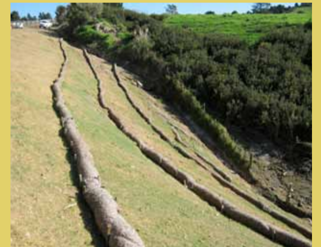
A series of Wattles installed as SIDs (slope intervention devices) slowing water velocity across the slope.
